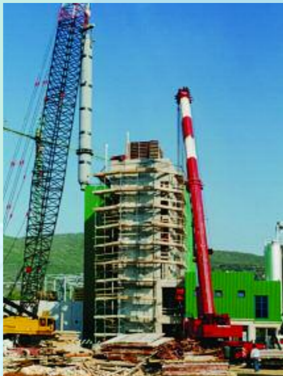
Coffee decaffeination plant Supplied under Schoeller- Bleckmann
