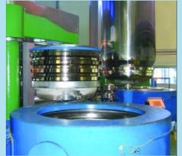
Edible oil extraction plant
