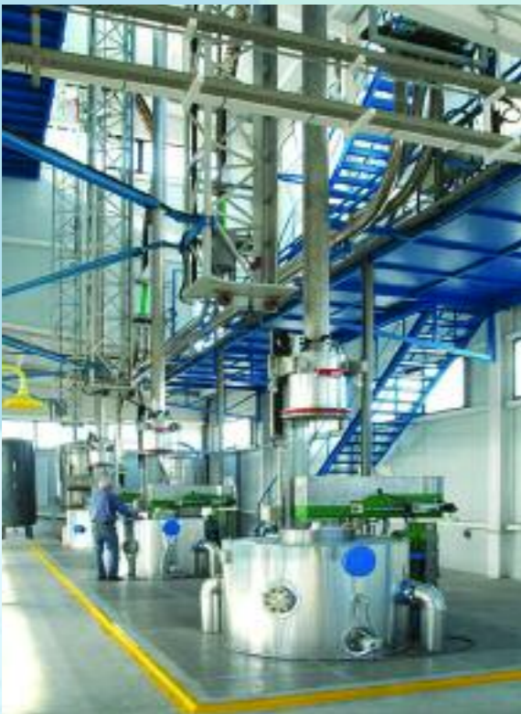
Cork purification plant
