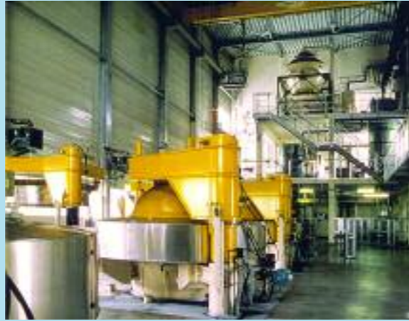
Tea decaffeination plant Supplied under Schoeller- Bleckmann
