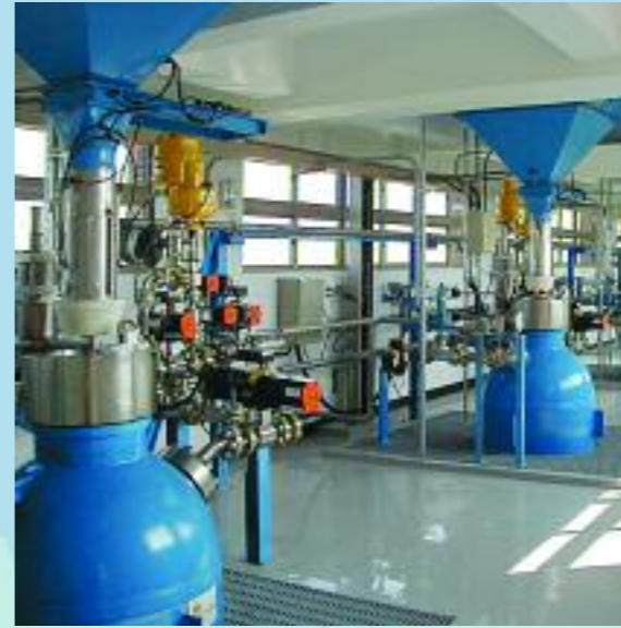
Rice treatment plant
